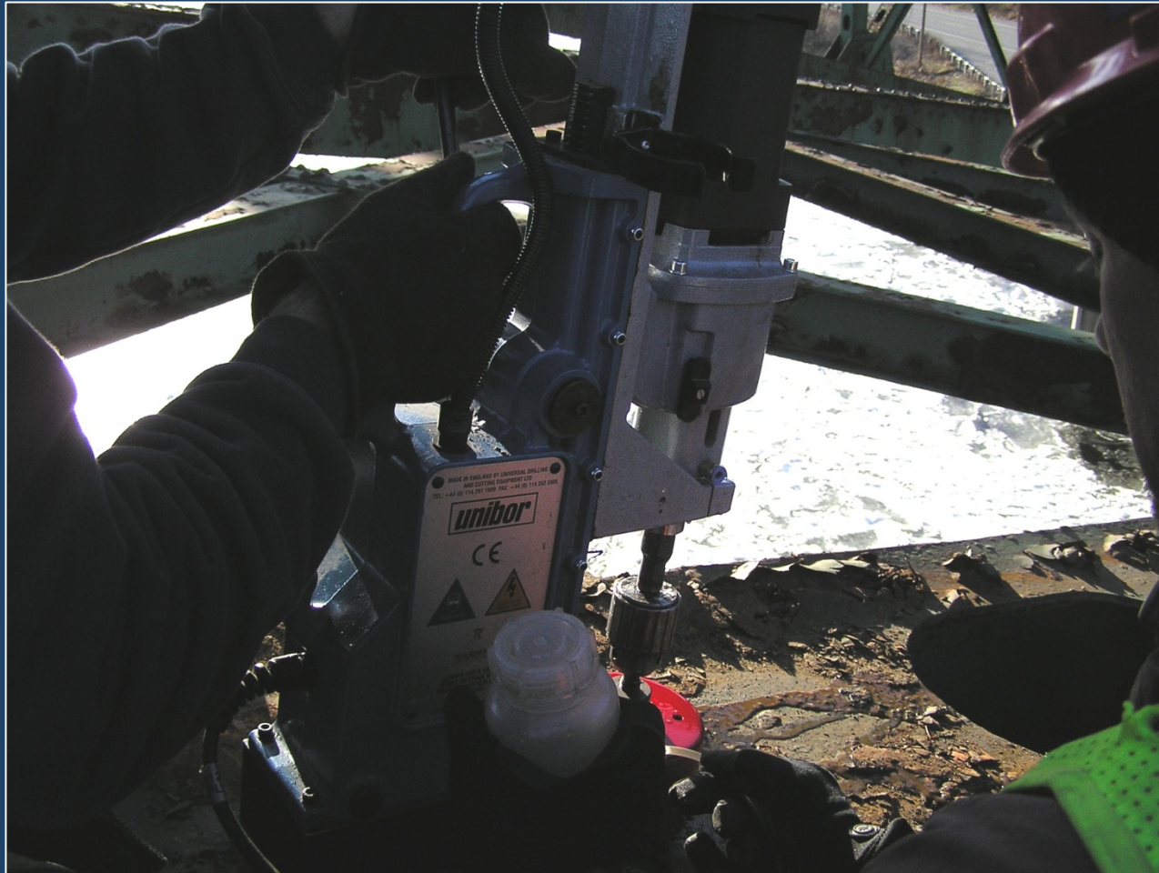
Coupon Extraction from Truss Cover Plate
